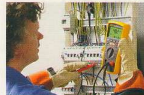
Insulation test at a distribution panel
